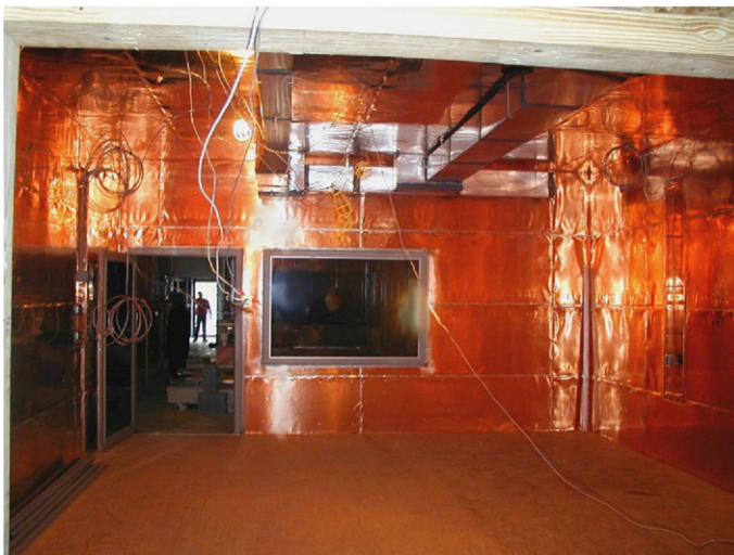
Figure 4. Photo showing the copper barrier applied before the installation of sheetrock, flooring, and ceiling tiles of an MRI suite.
